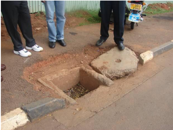
Picture 5: “Other Kampala Inner Roads” Dewinton Rd. Drainage blocked due to lack of Manhole covers. (Stirling/ KOM)
