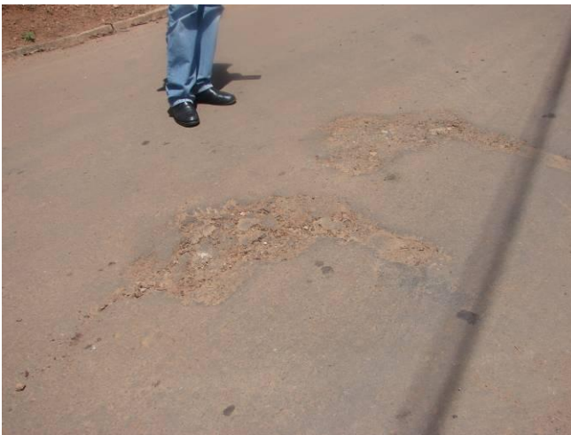
Picture 11: Road failure noted on the asphalt overlay on Elizabeth Road
