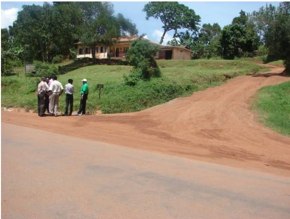
Picture 26: 2 nd sealing at road junctions. Salaama Rd. Note the silting. (Dott Services/ MBW)
