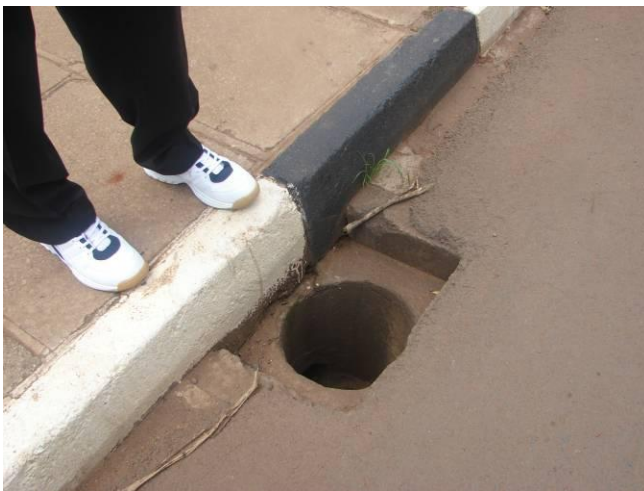
Picture 7: Steel Gratings missing, are dangerous to pedestrians and will cause blockage. Nile Avenue “Other Kampala Inner zone Rds - Stirling /KOM
