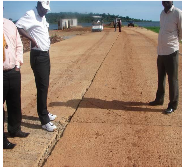
Picture 18: Casting concrete, expansion joints and installation of guardrails still on going. Munyonyo – Marina – Spencon/PROME
