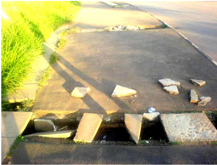
Picture 1: Pre-cast slabs near MoWT offices on Zana – Entebbe Rd. Note the poor quality of slabs due to lack of steel reinforcement. (EnergO/ MBW)
