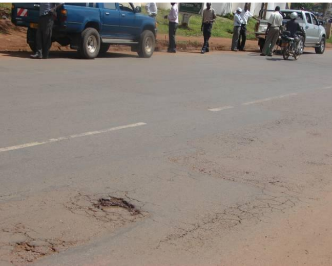
Picture 15: Failure of the patching . Jinja Rd near Lugogo Indoor Stadium. (Cementers/ PROME)
