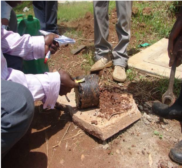
Picture 17: Measuring the thickness of the asphalt core. Jinja Rd near Lugogo Indoor Stadium. (Cementers/ PROME)
