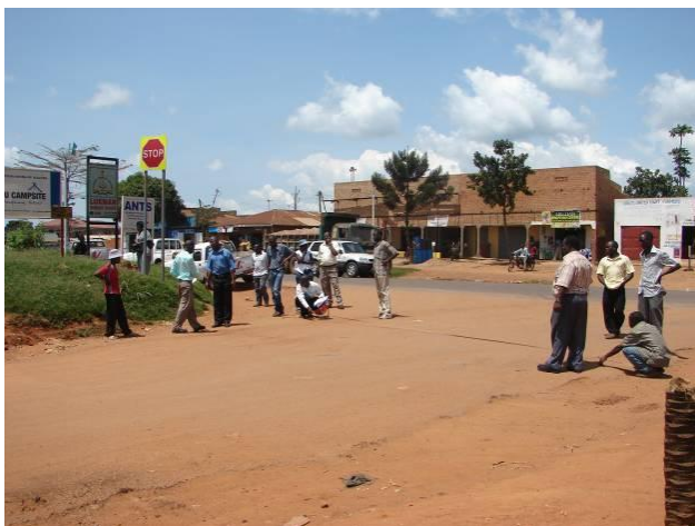
Picture 3: Measuring of junctions to ascertain surface dressing quantities on Zana - Entebbe Rd. (EnergO Ltd/ MBW)
