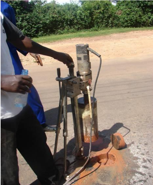
Picture 13: Coring to test asphalt quality and thickness on Prince Charles Drive. (Spenco/ PROME)
