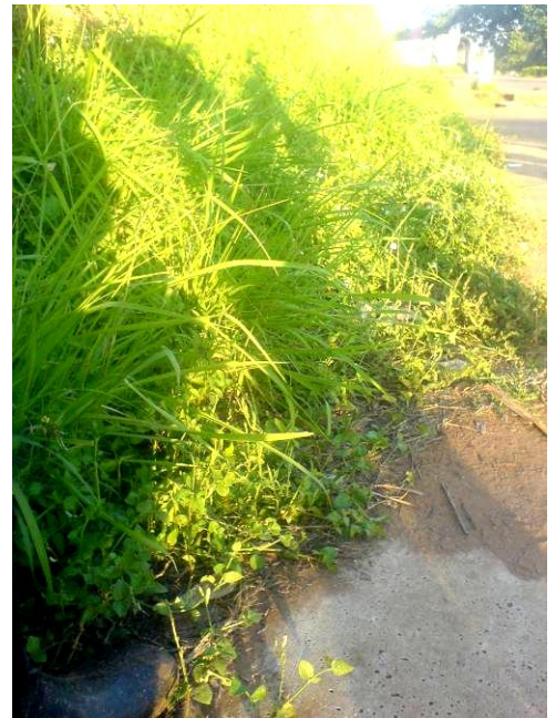
Picture 2: Pre-cast slabs near MoWT offices on Zana – Entebbe Rd could not be ascertained due to overgrown bush on top. (EnergO/ MBW)
