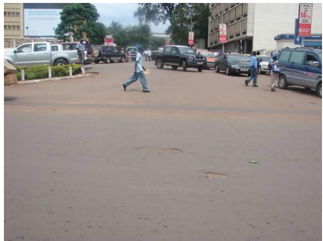
Picture 8: Road failure of the overlay on Kampala – Jinja Rd near the Junction to Embassy House - Stirling /KOM
