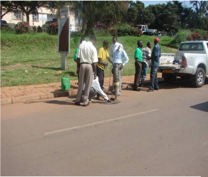
Picture 14: Coring to test asphalt concrete thickness and quality. Jinja Rd near Police Station. (Cementers/ PROME)
