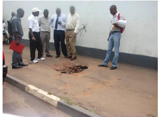
Picture 6: Pavement failure on the Walkways on Dewinton Road
