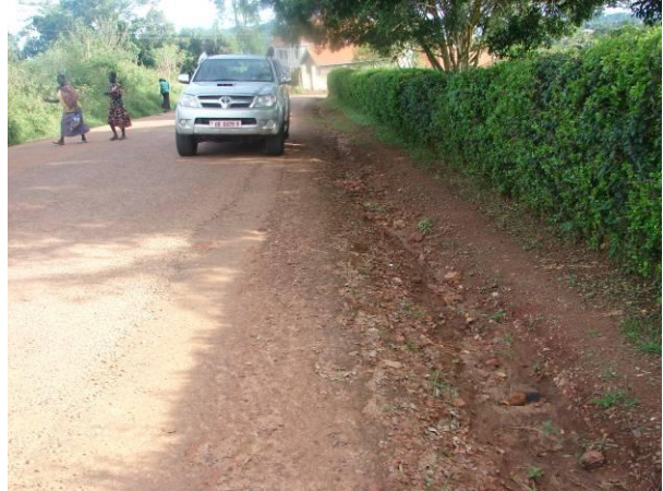
Picture 10: Lukuli – Buziga – Munyonyo Rd. lack of drainage intervention in the design scope. (Mulowoza/M&E Assoc.)
