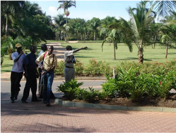
Picture 24: Munyonyo CWR driveway and parking. Verification of road Kerbs. (Dott Services/ MoWT)
