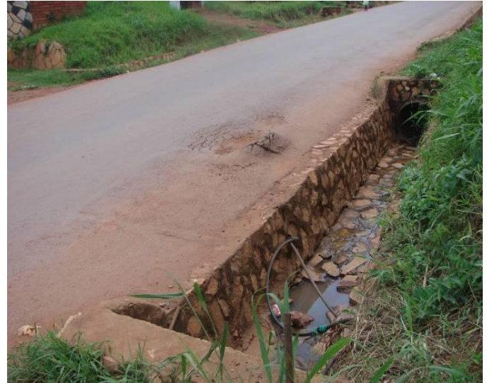
Picture 29: Road failure of asphalt concrete due to water connection leakage after road works. Kyadondo II (Dott/ KAGGA)
